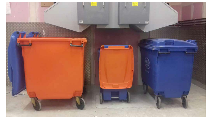
Figure 5.2: Chute system at Battersea Reach (credit: Hardall.co.uk)
