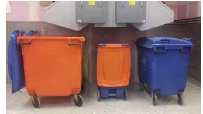
Figure 5.2: Chute system at Battersea Reach (credit: Hardall.co.uk)
