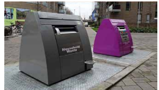
Figure 5.6. Underground waste collection system
