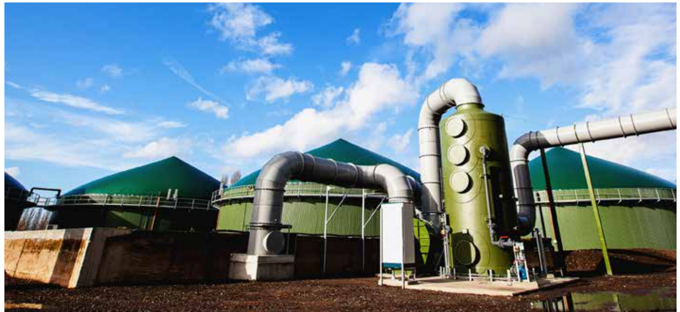
Figure 6.9: Coleshill food waste anaerobic digestion plant (credit: Severn Trent)
