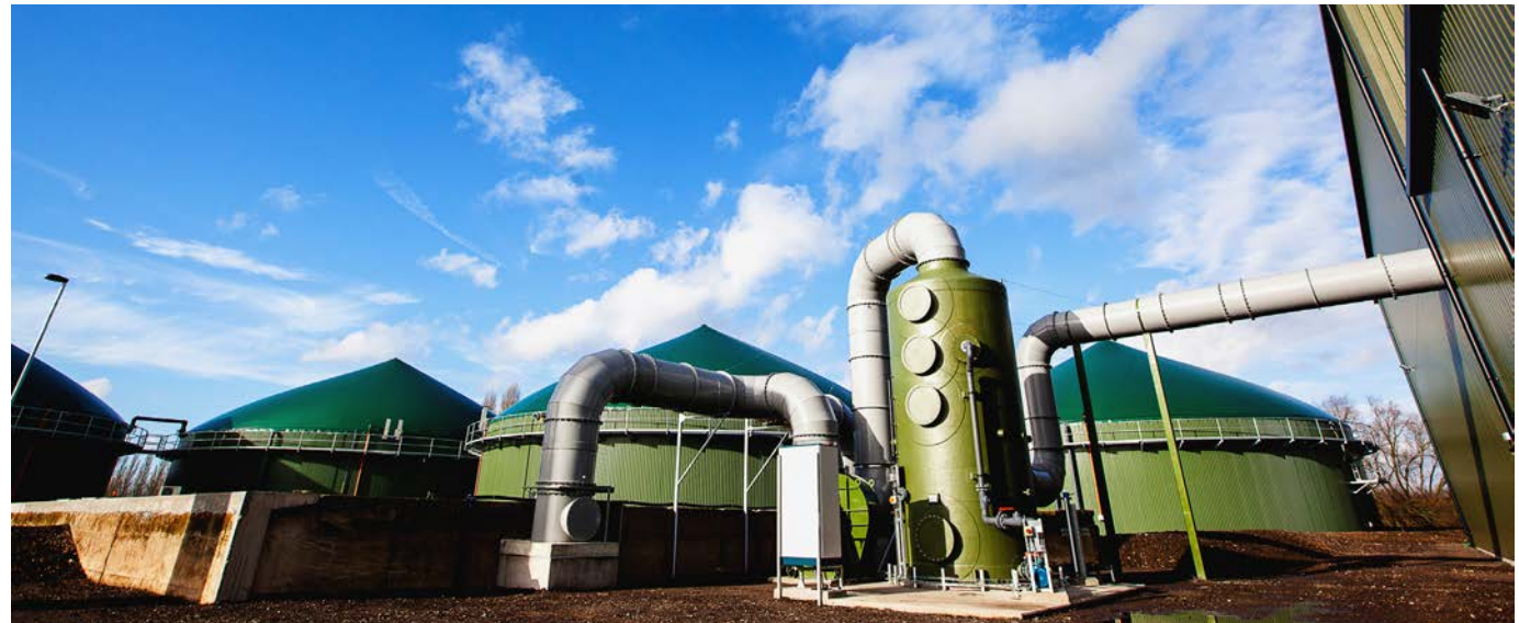
Figure 6.9: Coleshill food waste anaerobic digestion plant (credit: Severn Trent)
