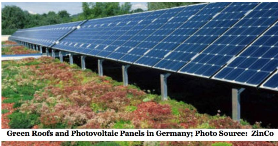
Figure 12. Co-existence of green roof and PV panels
