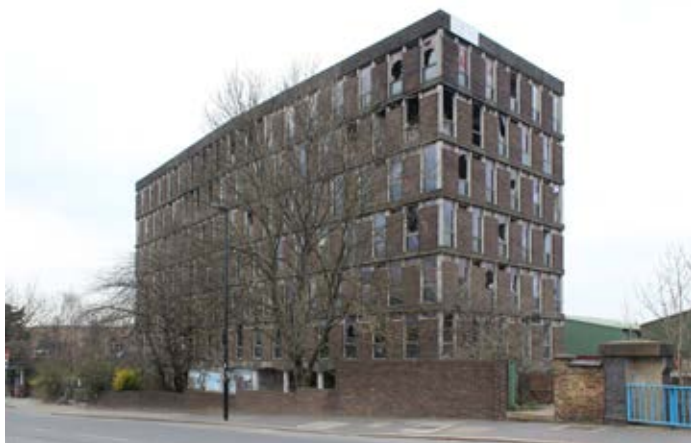
Figure 6: The derelict Wall's House (latterly Nash House), of c.1968 by Beard, Bennett, Wilkins & Partners. The canal bridge is at the right of the photograph (P6846003).
