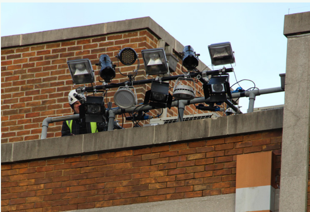
A contractor installs different types of lighting equipment onto theatrical lighting bars to demonstrate different light qualities and effects · Image: Speirs Major
