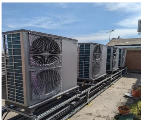
Figure 7: CREW Energy's heat pump installations at Devas Club
