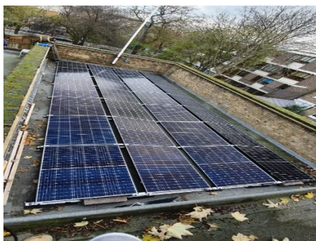
Figure 6: CREW Energy's solar panel installation at Islington Sea Cadets
