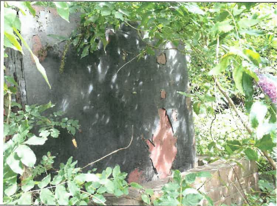
Photo 51: Building 3 – Oil tank to rear
