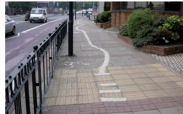
Figure 2.5.2: Current condition of cycle lanes on Nine Elms Lane.
