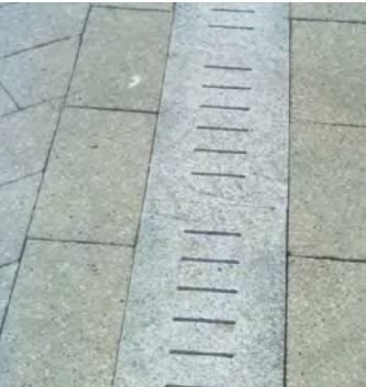
Discreet surface storm water
