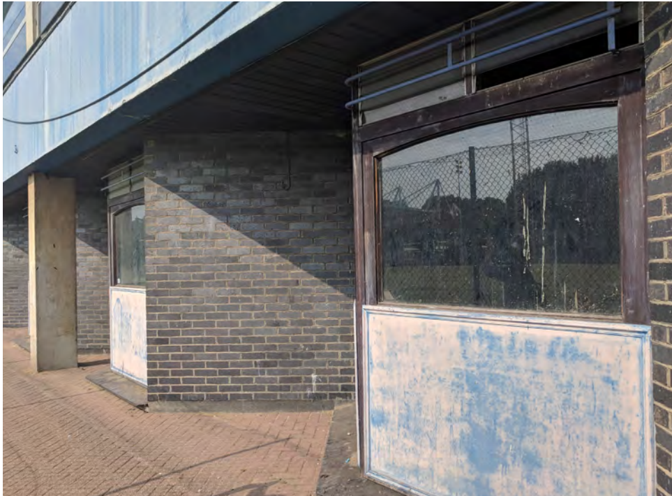
10. Bar building in disrepair and unused.
