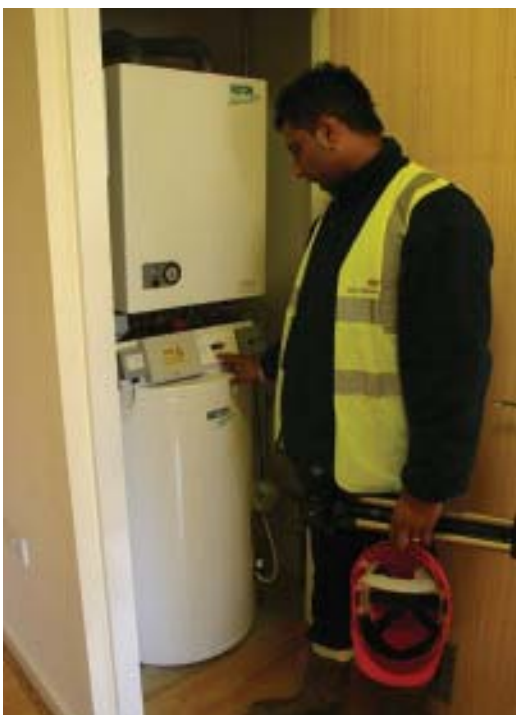
The boiler room at Grand Union Village (left).
