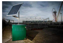
Fuel cell & solar powered lighting for construction at the Olympic park
