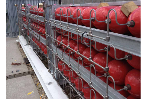
Hydrogen storage (compressed gas)
