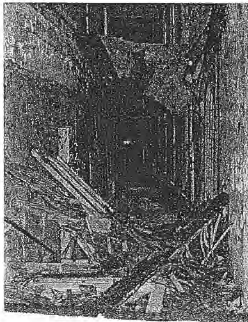
04 Collapsed upper floor due to water ingress
