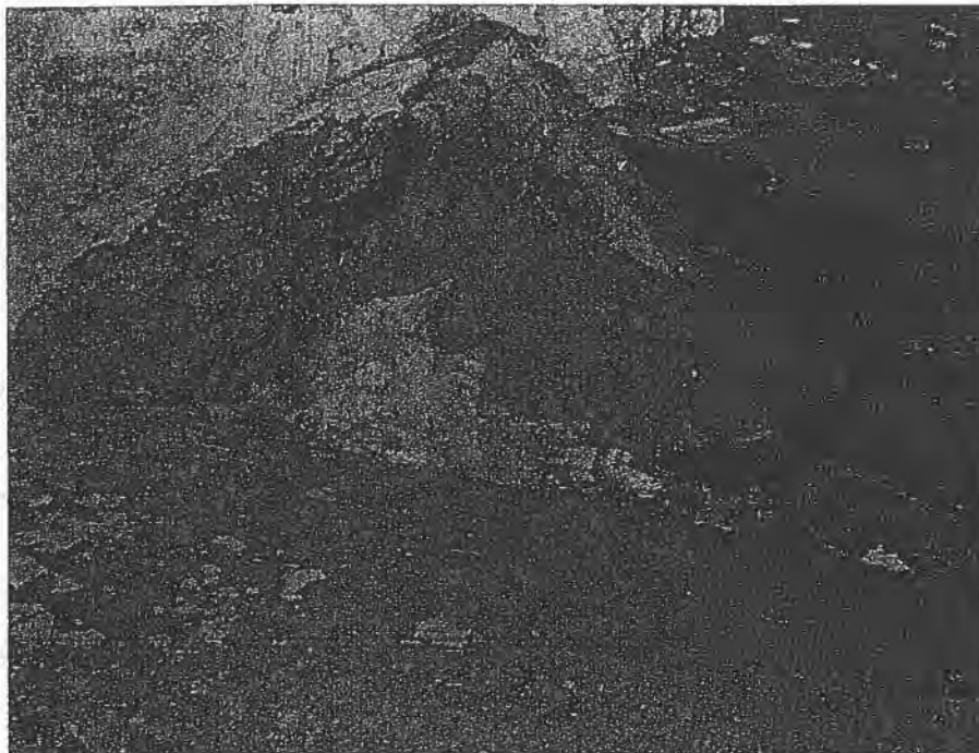
07 Failure of floor of 6A
