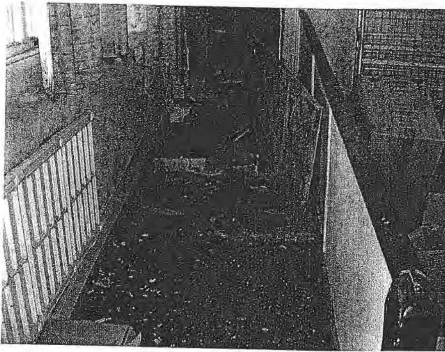
09 Damage to Floor
