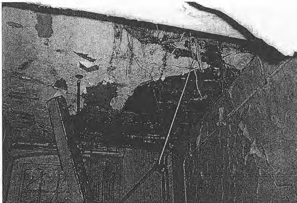
19 Rot to ceiling to Building C
