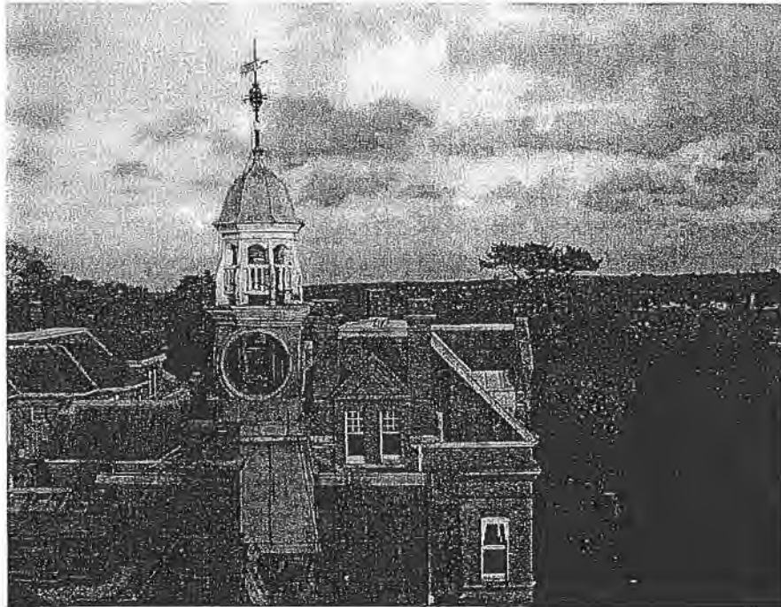
03 Clock Tower & Failing Lead Detailing
