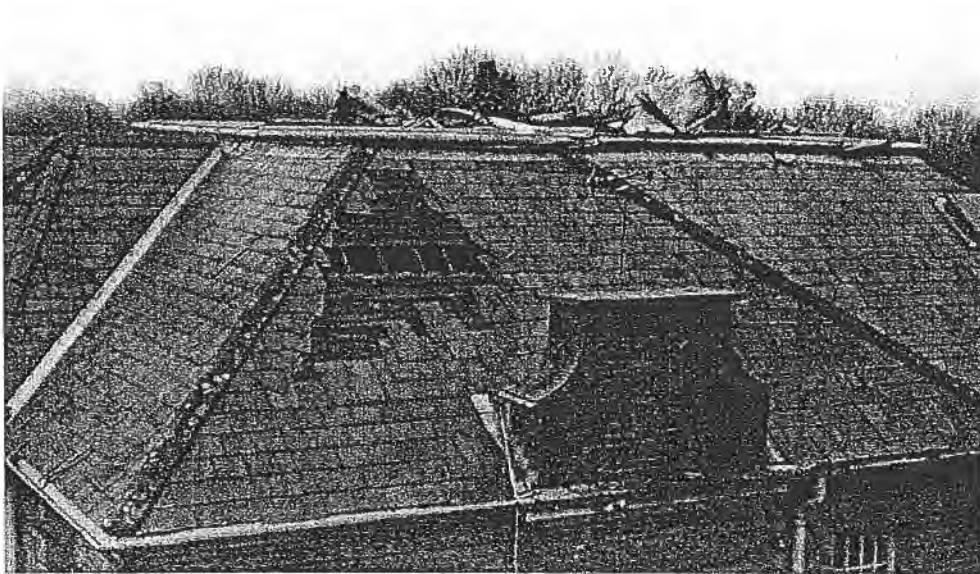
02. Vandalism to roof coverings
