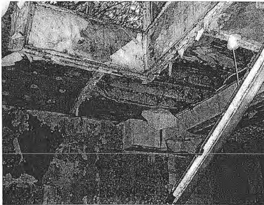
09 Failure of ceilings to 9A
