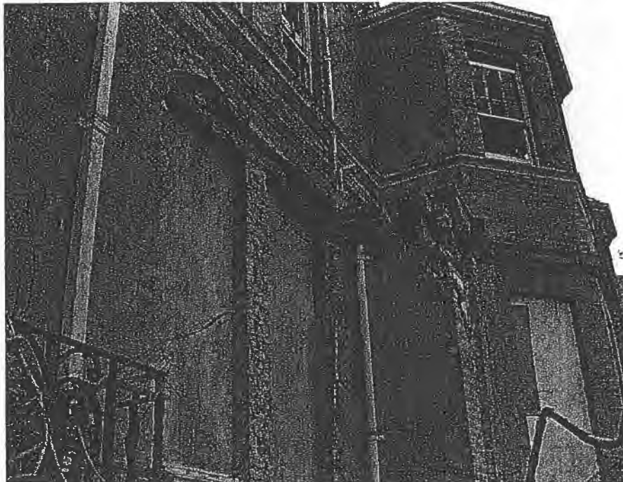
06 Structural Damage to East Wing
