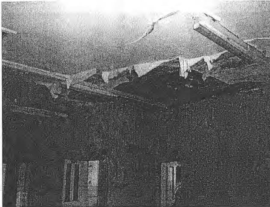
07 Water ingress through ceilings in 14A
