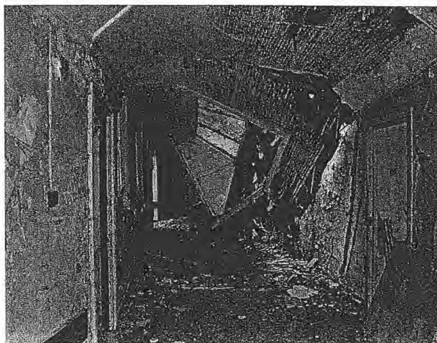
10 Collapse of roof structure to corridor
