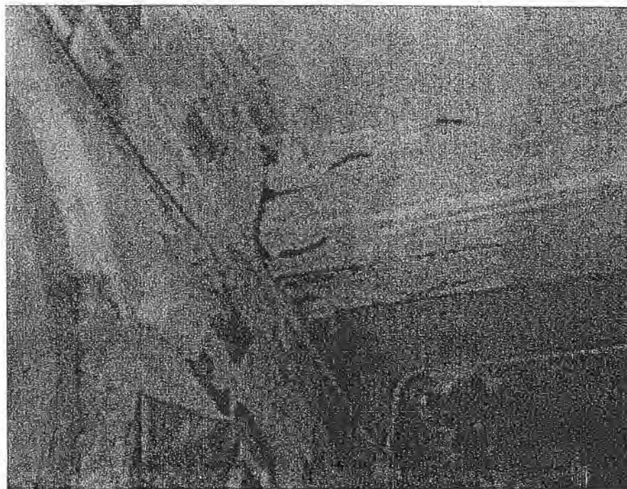
09 Rot decay to end of timber beam
