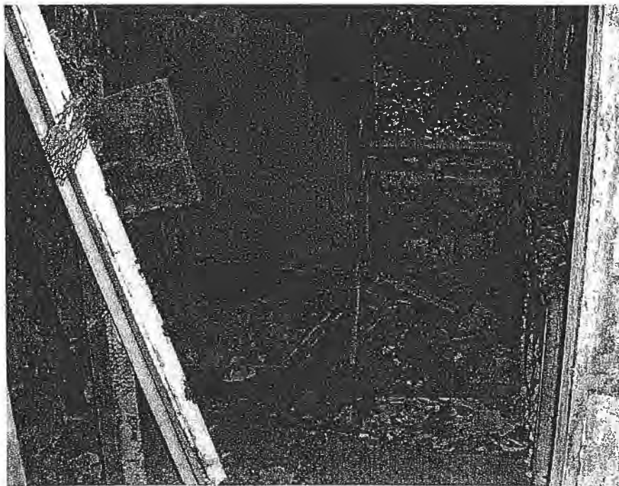
08 Damage to Ground Floor
