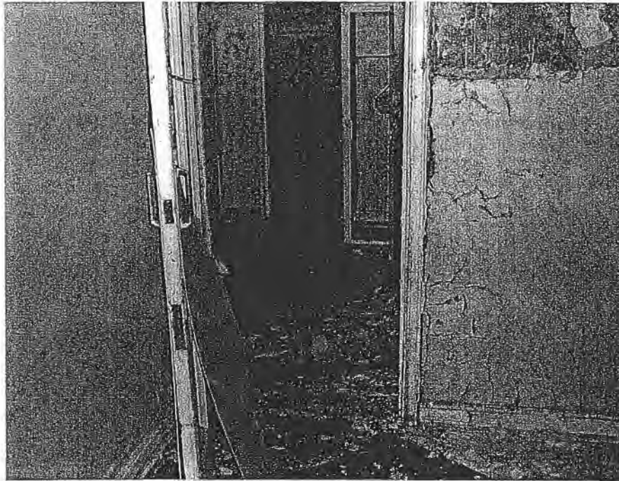
07. Collapsed timber floor
