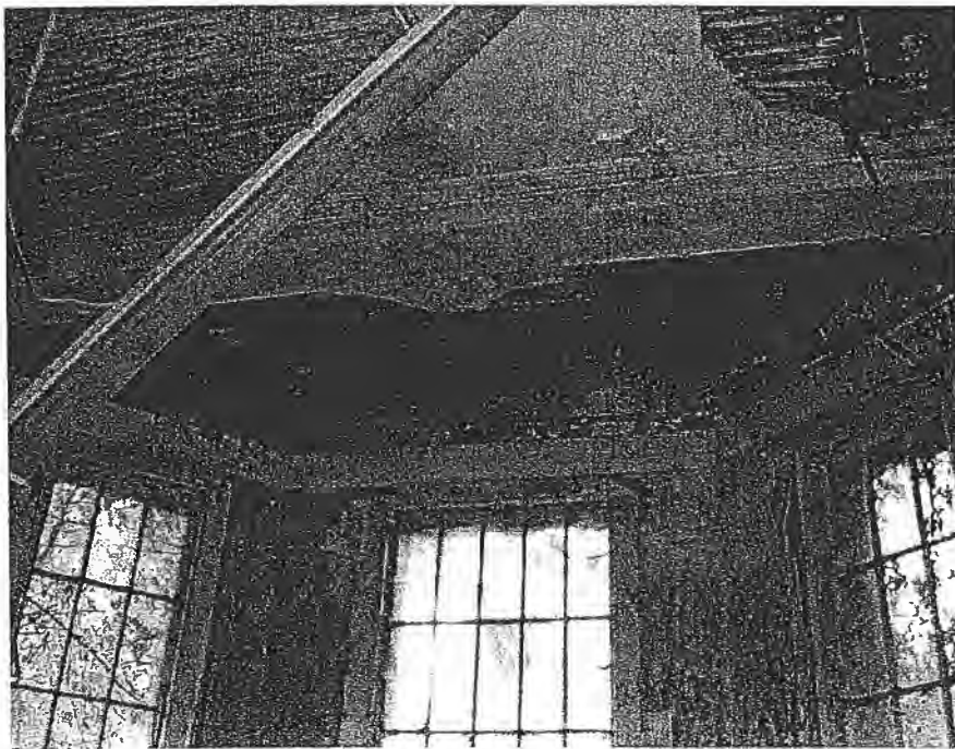
10 Damage to ceiling and walls below bay roof
