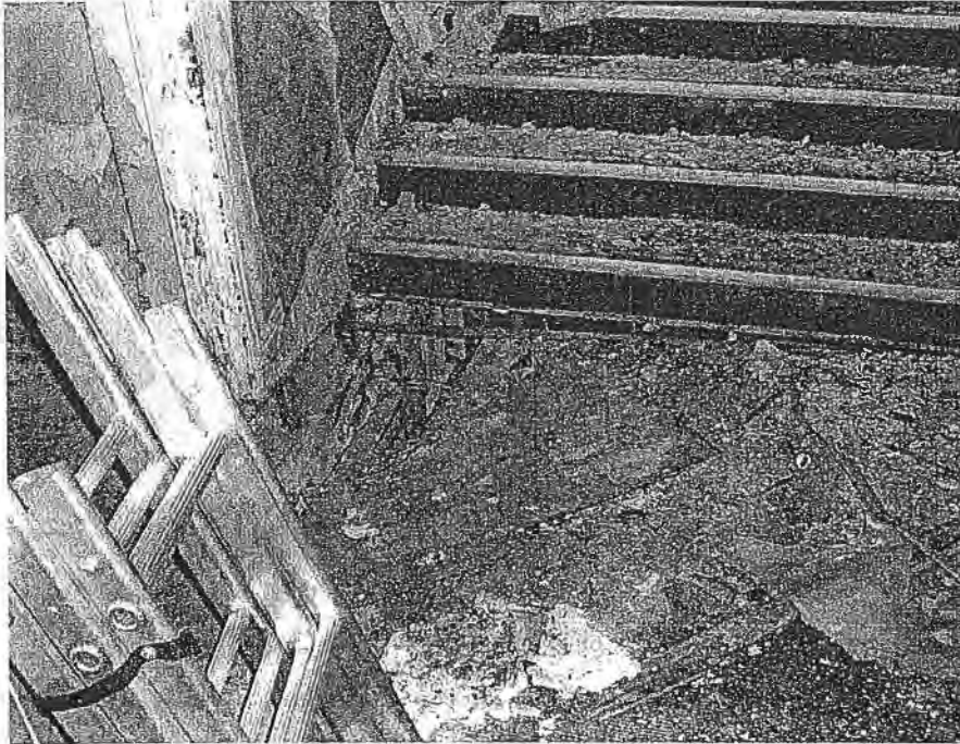
09 Decay to floor due to water ingress
