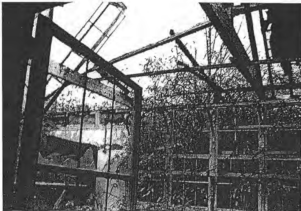
08. Fire damaged corridor
