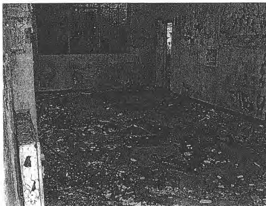
12 Condition of floor in parts of 19B
