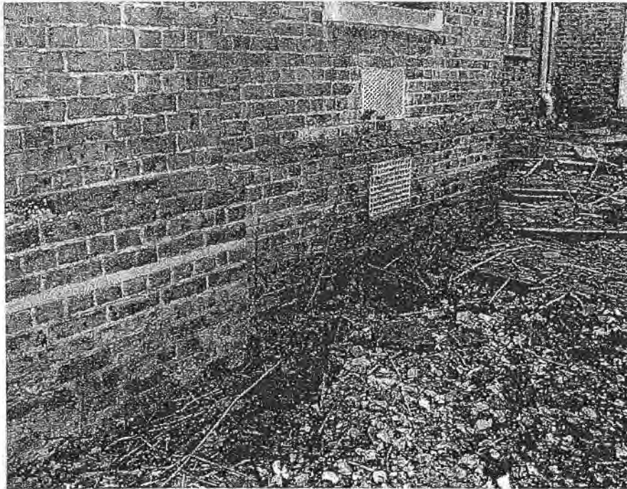
11 Spalling brickwork to 20B
