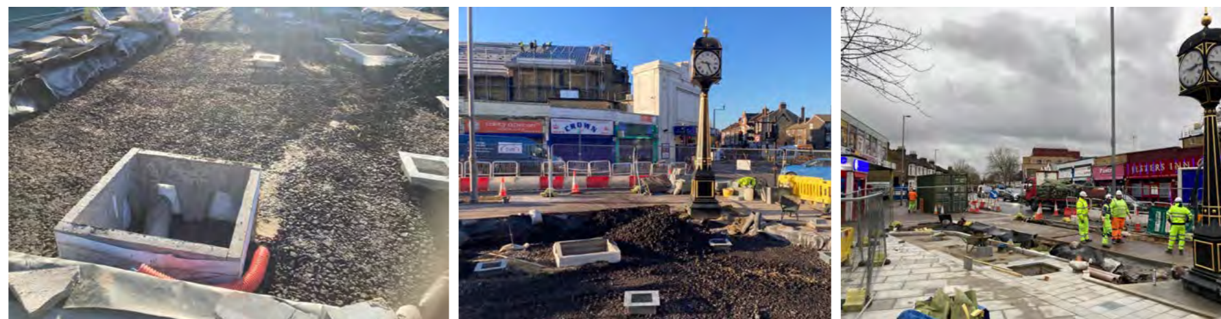
Figure 57: Construction works at Markhouse Corner, London Borough of Waltham Forest [credit: London Borough of Waltham Forest]
