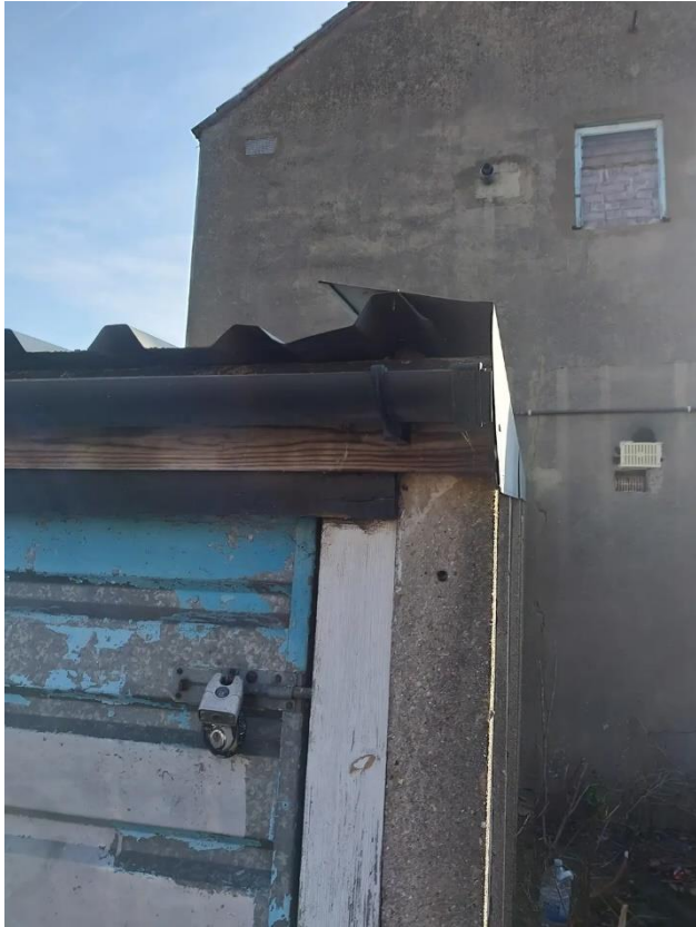
Plate 3.3 Left (TN3) a small crevice between roofing tin.
