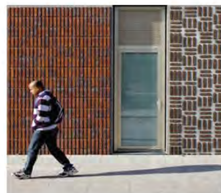
✗ Fig. 159. Incoherent mix of different brick coursing and colours
