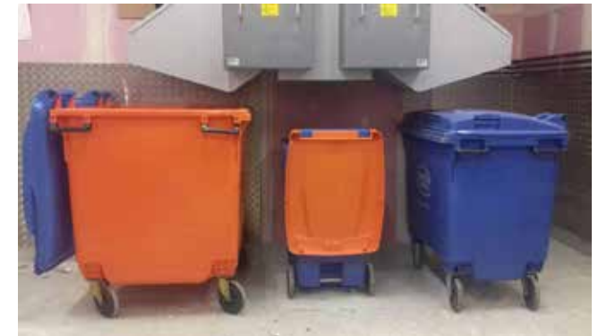
Figure 5.2: Chute system at Battersea Reach (credit: Hardall.co.uk)
