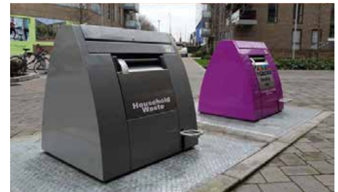
Figure 5.6. Underground waste collection system
