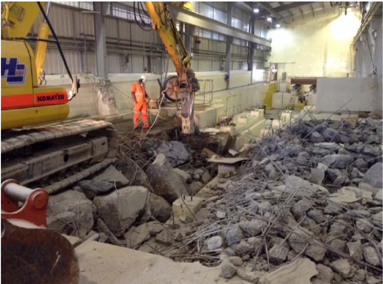
Wheel lathe break-out at New Cross Gate Depot
