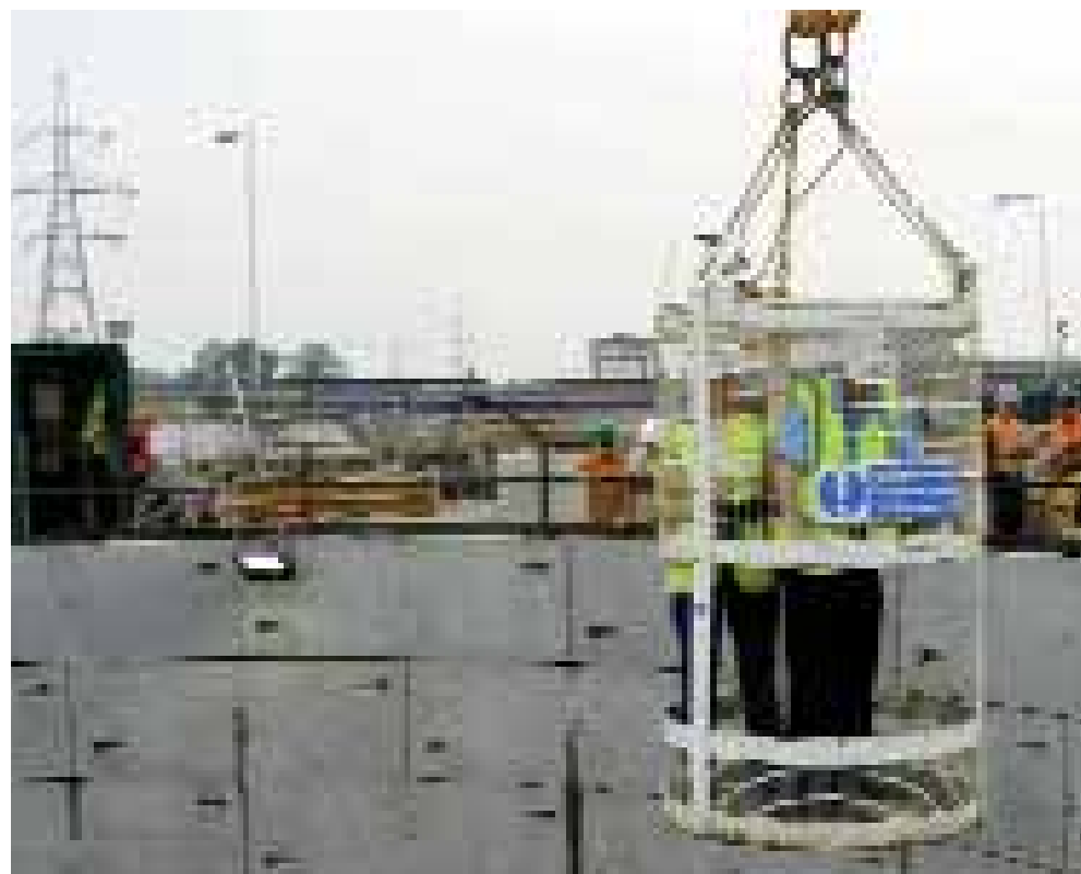
A huge tunnelling project is taking place on the Olympic Park site to bury the powerlines which currently scar the landscape.
