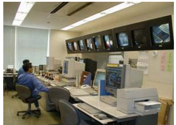
Control room / Chiba
