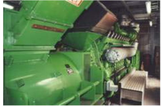
Gas engine 1.5 MW / Chiba
