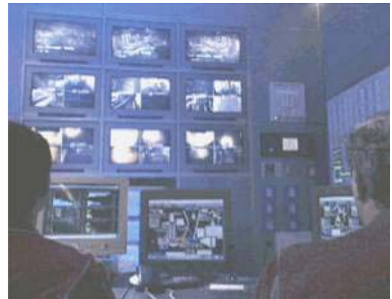
Control room / Karlsruhe
